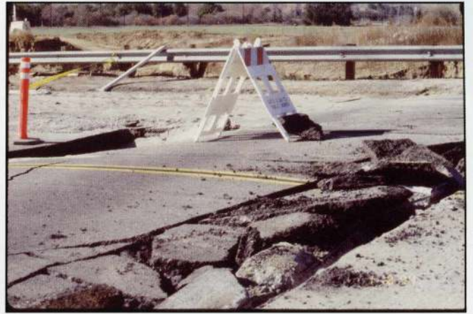
Local roads were severely damaged as a result of the 1994 Northridge earthquake.
