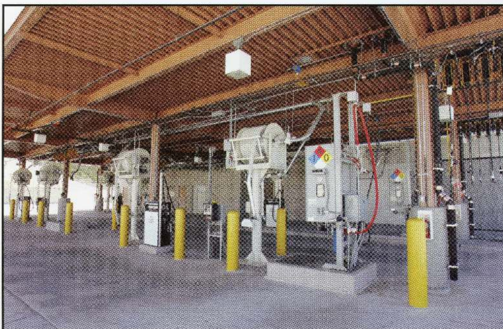
The Transit Maintenance Facility in the Valencia Industrial Center opened in 2006 and provides a central location for the City's transit fleet. Pictured here: bus wash area.
