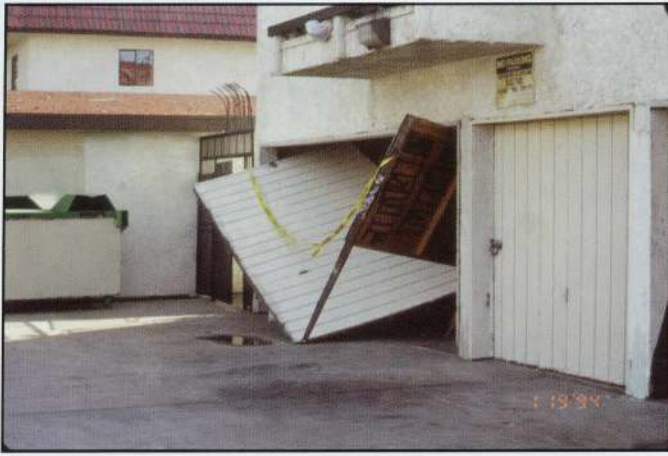
Many people were forced to evacuate their homes because of earthquake damage.
