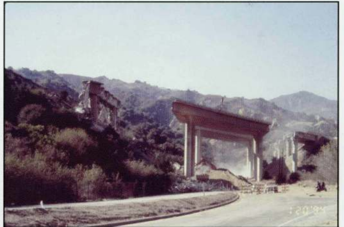
The earthquake caused millions of dollars in damage to local roads and freeways. Pictured here is the collapse of a bridge along Interstate 5 in the Santa Clarita Valley.
