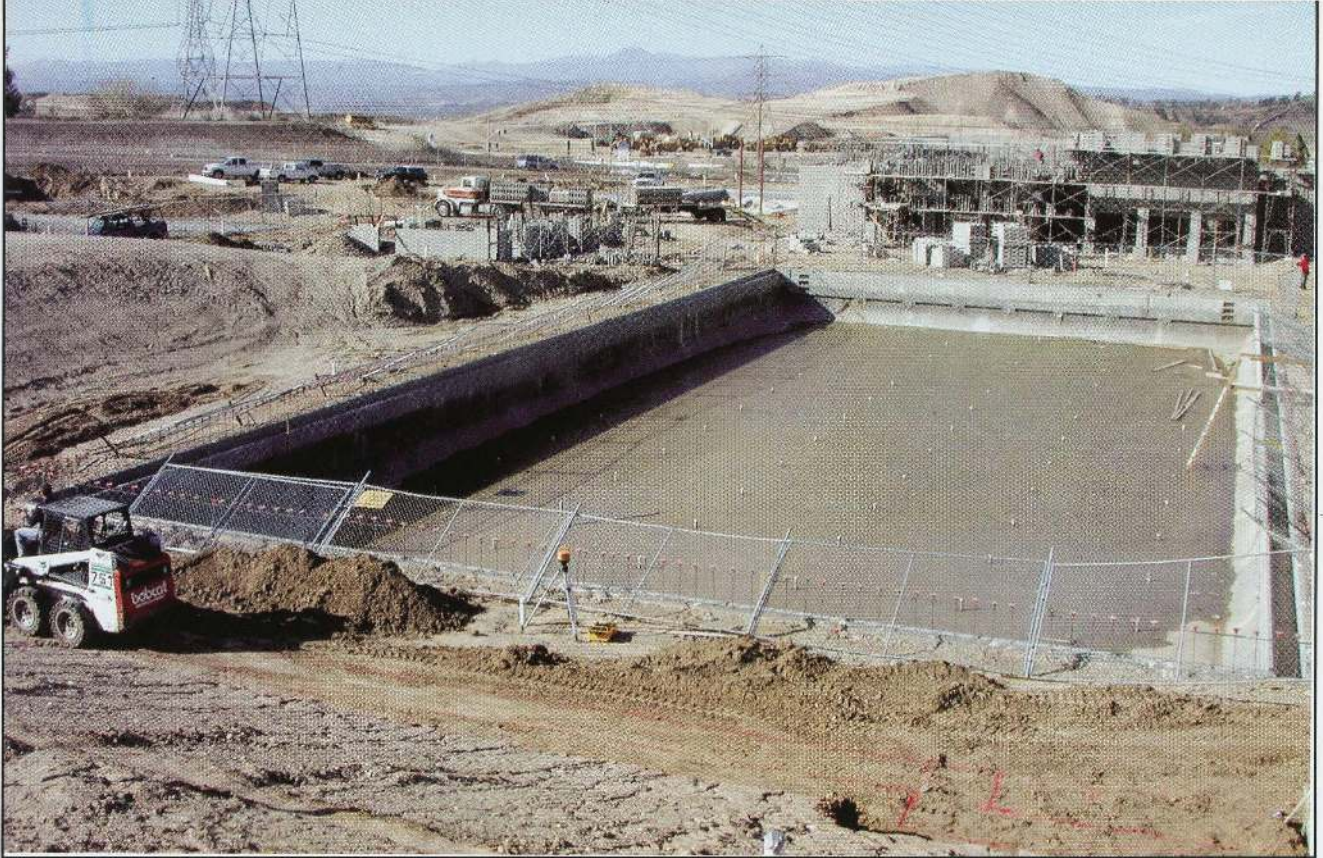
The City's Aquatic Center at the Santa Clarita Sports Complex under construction in early 2003.
