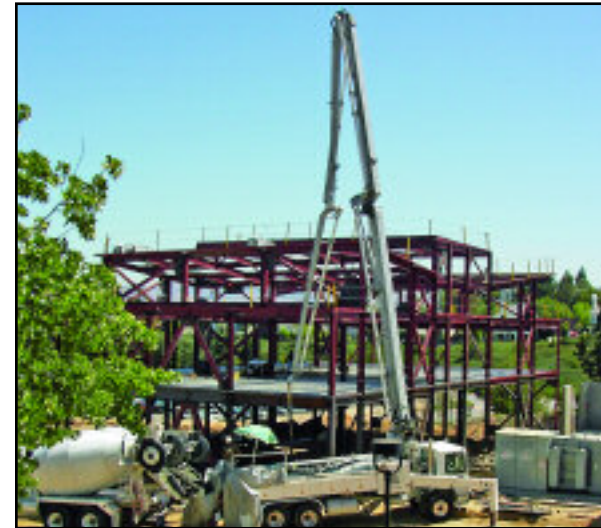
The Music Dance Building begins to rise next door to the Vital Express Center for the Performing Arts in mid-2004.
