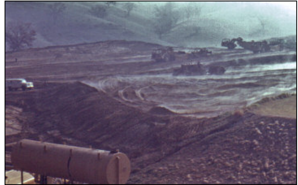
The hills south of Valencia Boulevard are graded to prepare for the construction of permanent campus buildings. The clattering steel behemoths kicked up an endless supply of dirt and dust at the nearby temporary campus.
