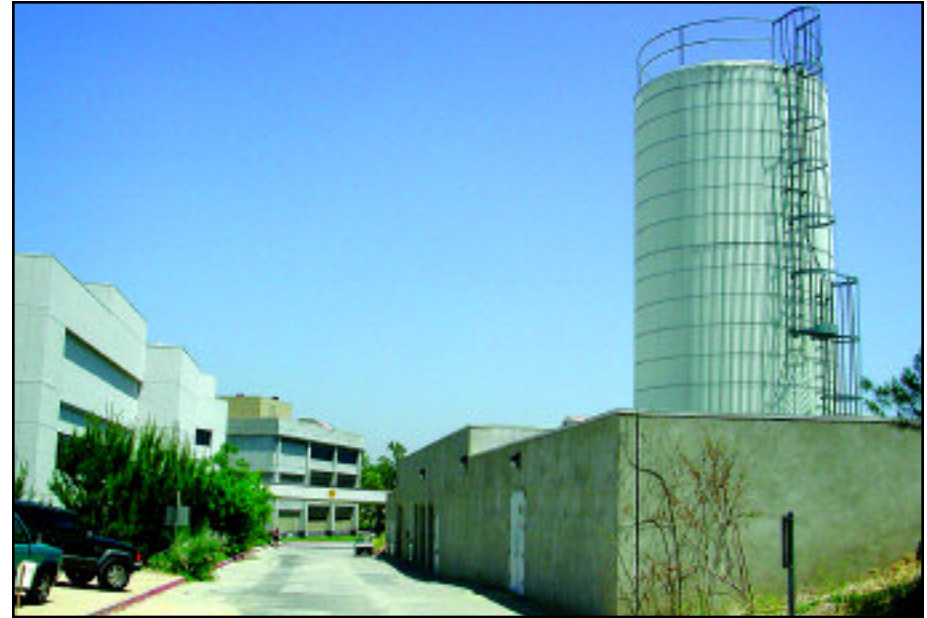
The Central Plant (above) was built to provide heating and air conditioning to two new buildings: the Media & Fine Arts Building and the Library. Its efficiency resulted in a 25 percent savings in energy costs.
