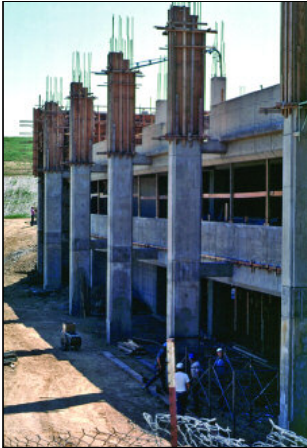
The Instructional Resource Center begins to take shape, having risen two of its eventual four stories.
