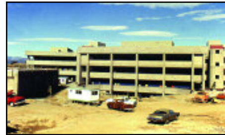
The Student Center (top) and, beyond that, Cougar Stadium are under construction. Most of the Instructional Resource Center (above) has been completed. This view is from the south. Just beyond the trailer is the present-day Bonelli Amphitheater.
