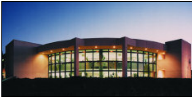
Most of the steel framework (top) has been erected for the new library (above).
