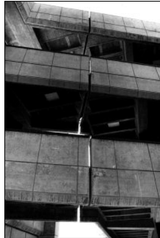
This expansion joint where the IRC and C Building meet was widened from the force of the 1994 quake.
