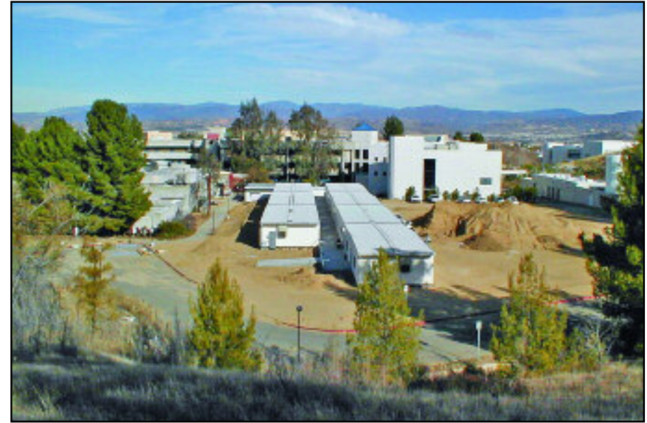
The Modular Classroom Village provided about 10,000 additional square feet of much-needed classroom space for the crowded campus.
