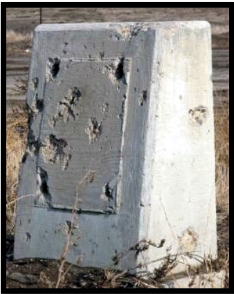
Figure 38: The monument shown on the map above. The interpretive marker is missing.
