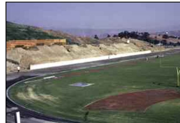
A crane hoists a bank of lights into place at Cougar Stadium, which itself is under construction (top). An earlier photo (above) shows the field, running track and a mound of dirt that was used as the foundation for the stadium.
