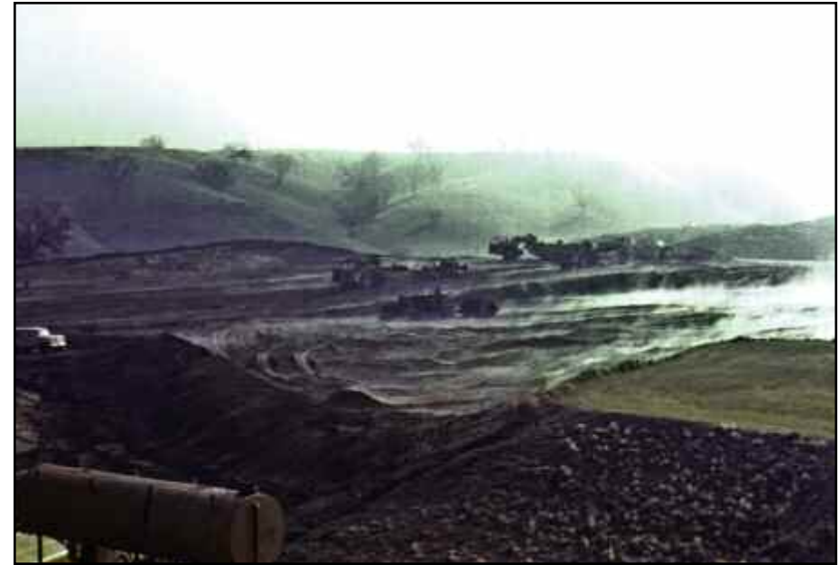
The hills south of Valencia Boulevard are graded to prepare for the construction of permanent campus buildings. The clattering steel behemoths kicked up an endless supply of dirt and dust at the nearby temporary campus.
