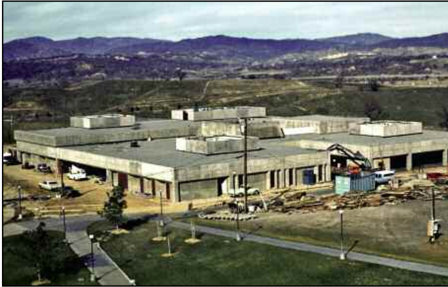
The Student Center (S Building) is under construction in this view looking north.
