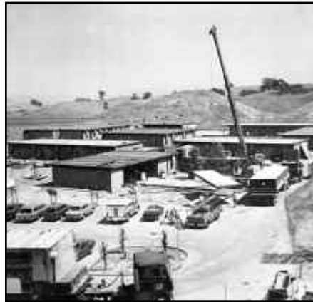
The athletic field, minus the stadium (top,) and the modular buildings (above) being erected to create the temporary campus.
