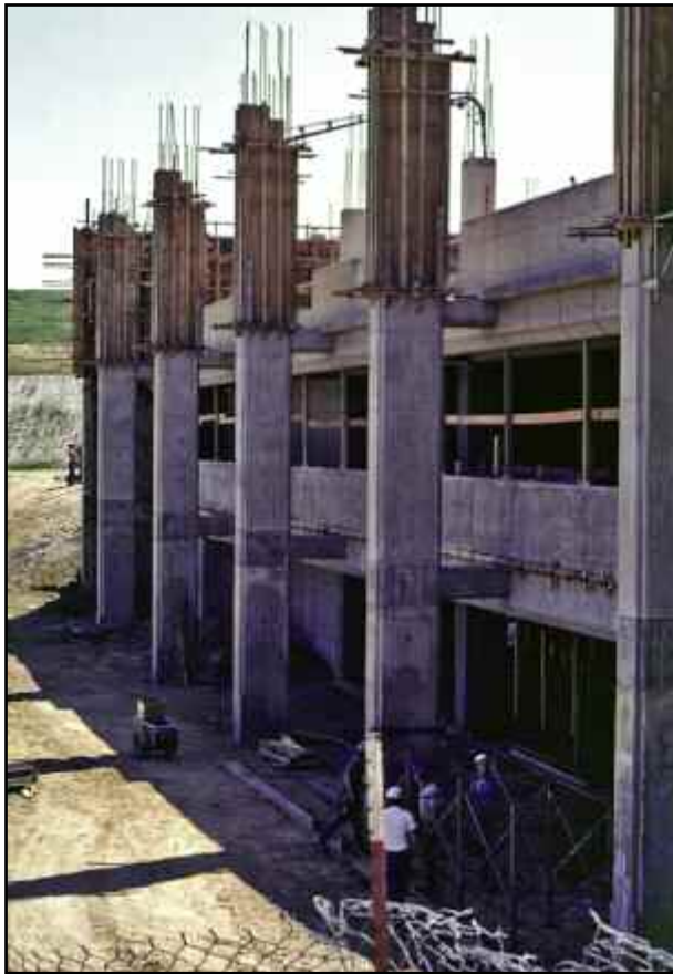
The Instructional Resource Center (Bonelli Hall) begins to take shape, having risen two of its eventual four stories.
