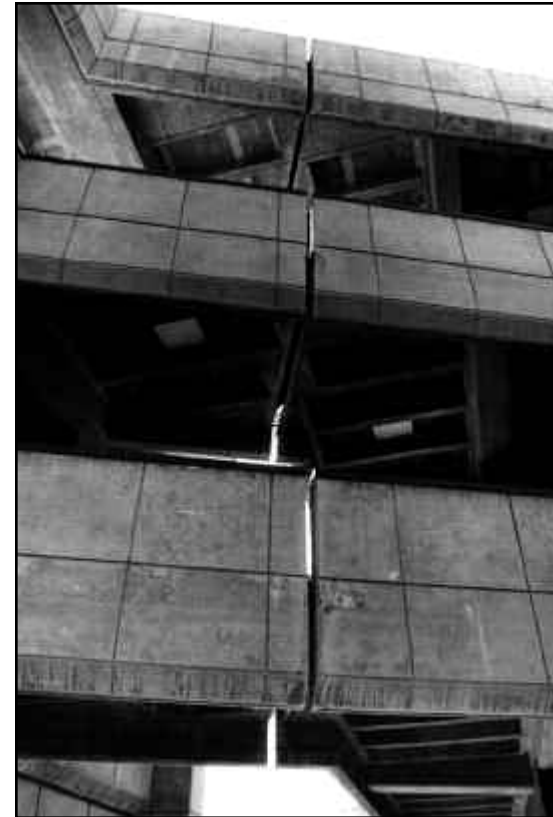
This expansion joint where the IRC (Bonelli Hall) and C Building (Seco Hall) meet was widened from the force of the 1994 quake.
