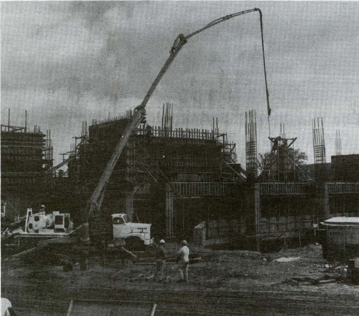
A hydraulic concrete pump with a 110-foot boom, reputedly the only one of its kind, is pumping concrete into the third-floor columns and walls of the William G. Bonelli Instructional Resource Center under construction on the south campus. The pump lifts concrete through the boom at the rate of 60 cubic yards an hour, saving many man-hours over more conventional systems. Engineers are hopeful of pouring the last floor in the four-story structure by the end of April.
