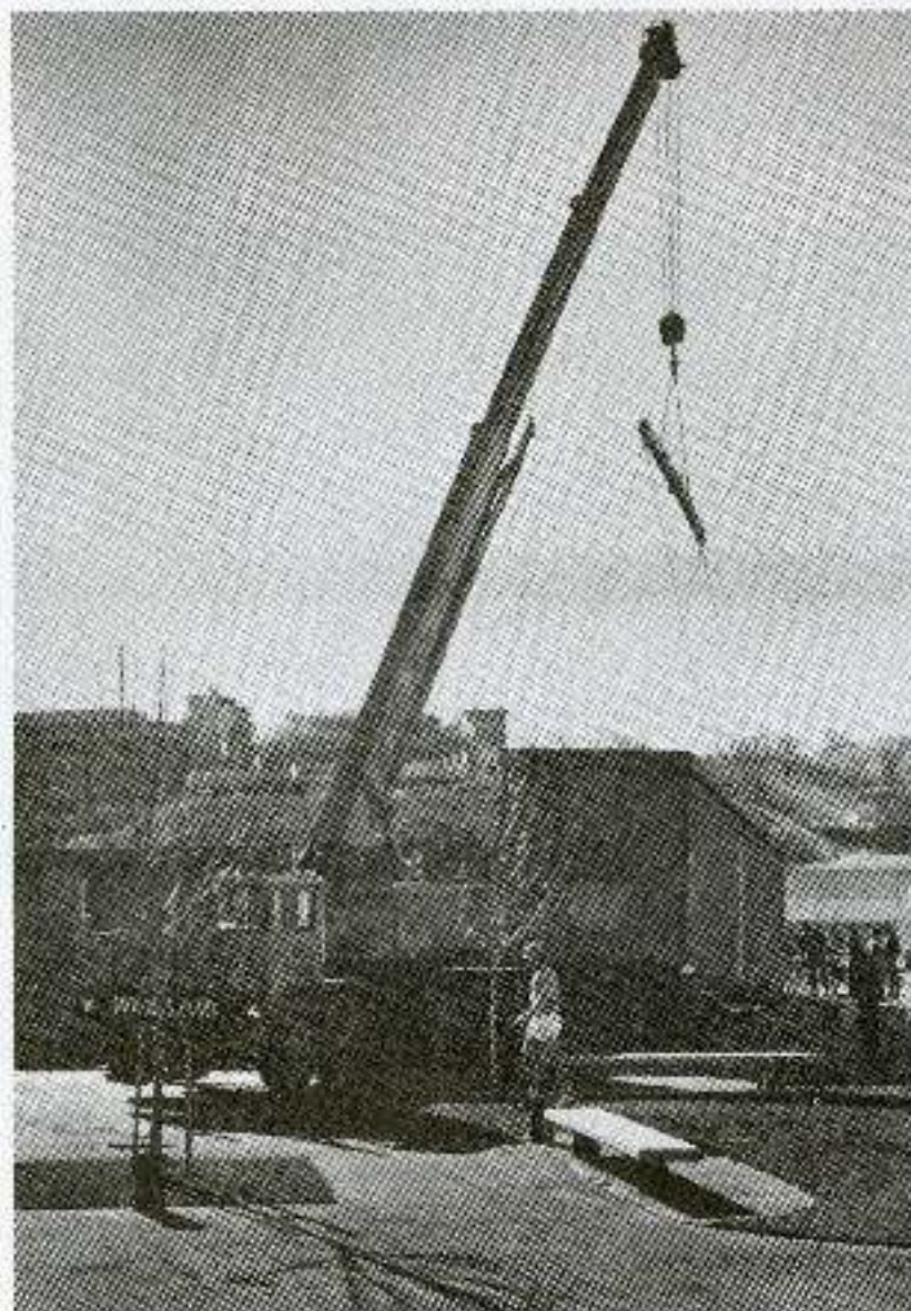
An era (the "Stag 13" period) is ending at COC as portable structures that served as classrooms and office for several years are moved out. In background are new Bonelli Center and the Laboratory building, the latter still under construction.
