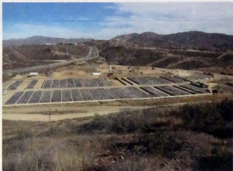
Soil treatment compound and treatment cells for bio-treatment of perchlorate
