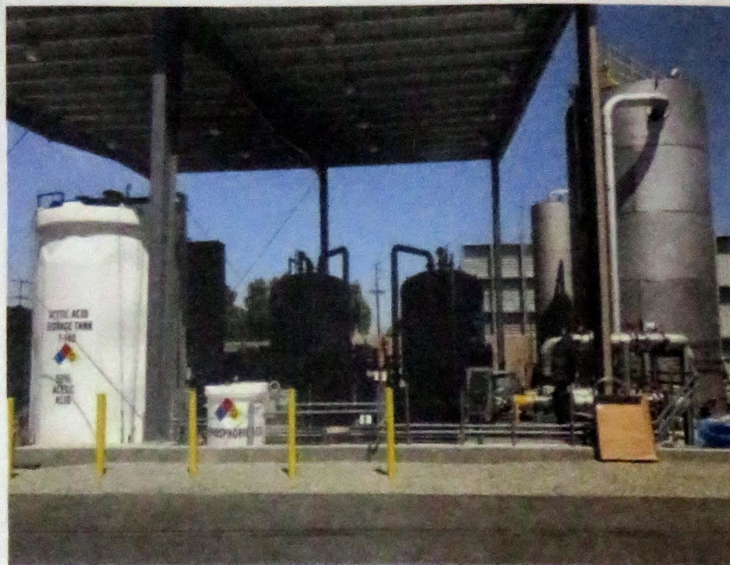
Groundwater treatment facility
