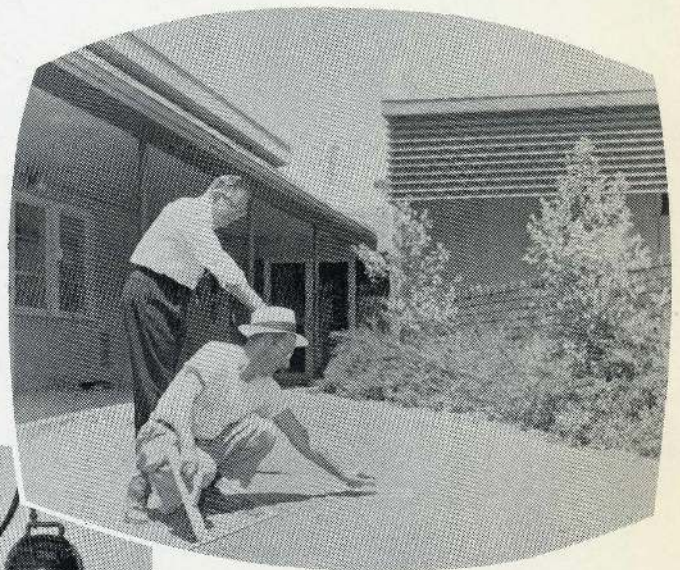
Inspector Edgar Bligh checks one of the many sections of concrete Mr. Charles Hipes troweled during the summer months.
