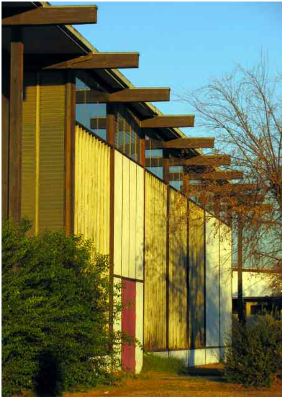
The City of West Covina relied on flawed cultural resource evaluations in approving the demolition of the 1959 St. Martha's Episcopal Church. Photo by Alan Hess.
