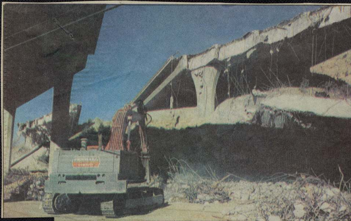
Workers continue to remove parts of the collapsed Antelope Valley Freeway connector ramp Friday. Detours around the severed junction are expected to be in place next week.
